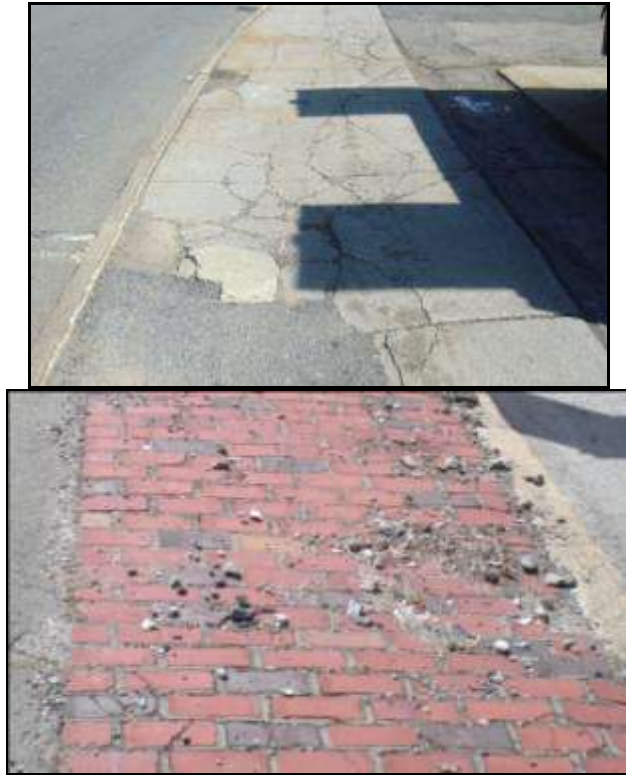
Figure 5: Cracked Sidewalk (left); Poorly maintained brick (right)
