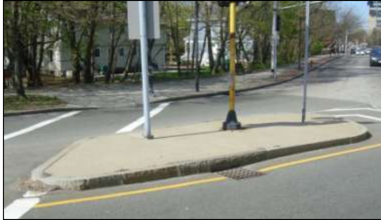
Figure 5: Inaccessible Walking button at Centre Avenue and Park Street
